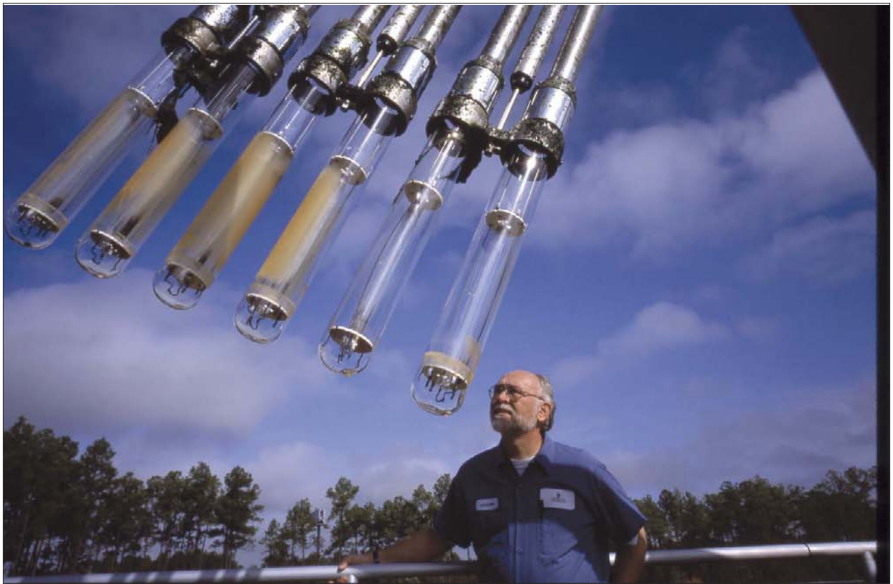
Above —Industrial photography is fun photography. One of my favorite annual reports was done for Southwest Water Company of Los Angeles. They build and run water treatment and waste water treatment facilities across the United States. This image shows UV lamps raised for cleaning. The UV from the lamps kills bacteria.
