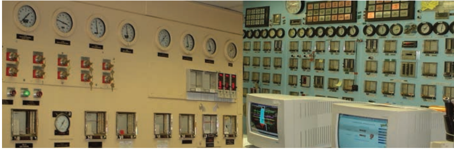
FIGURE 1.2 1950s pneumatic control panels.
