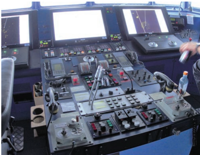
FIGURE 10.1 Example of an multivendor ship bridge systems (MBS) centre console of a contemporary patrol vessel.
